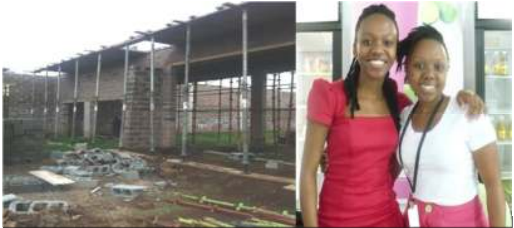
Frutee Belliez entrepreneurs Masibonga and Mbali alongside the construction site that is now their new factory in Waterfall, eThekweni. The enterprise's core business is preparation and packaging of vegetables and fruit.
